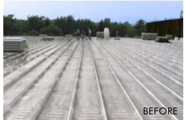
End laps, exposed fasteners, & penetrations caused this metal roof to fail.
